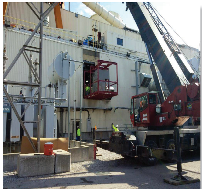
Figure 2 - Loading the new DECS-2100 into the facility
